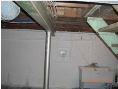
Plumbing along wall
